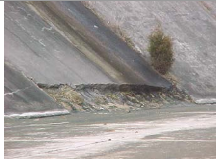
Spalled area, 40 feet long and 6 inches deep, 200 feet downstream of control section
