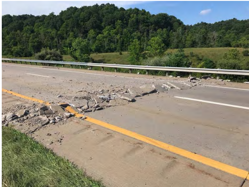
Figure 2.15.i – Road Buckling due to Heat on I-77, Noble County
