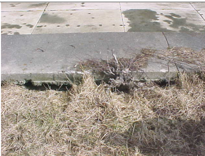
Void under top of slab, 400 feet downstream of control section
