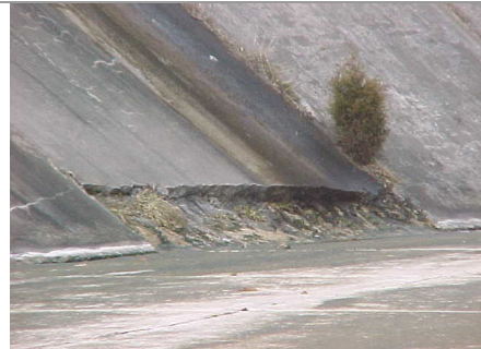
Spalled area, 40 feet long and 6 inches deep, 200 feet downstream of control section
