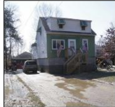
Murray Road Property – Photo taken following February 28, 2011 flood event. Notice the high water mark.
