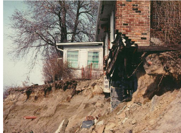
Damage caused by an eroding bluff in Cuyahoga County (1986).
