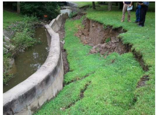
Damage from streambank erosion in the City of Pepper Pike.
