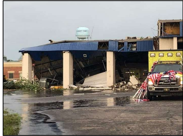
Damage sustained to Fire Department Facility
