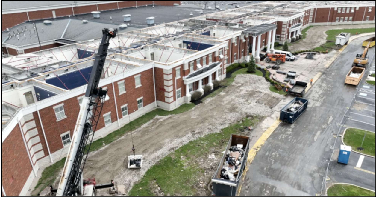
Lakeside High School in Saybrook Township, roof collapse – December 1, 2024
